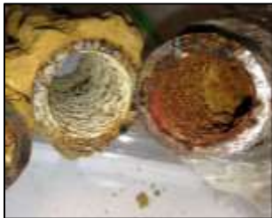
Corroded pipes from Flint. (Virginia Tech Magazine)
